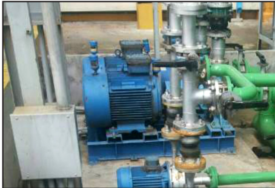
Inconsistent re-lubrication was contributing to motor bearing failure.
