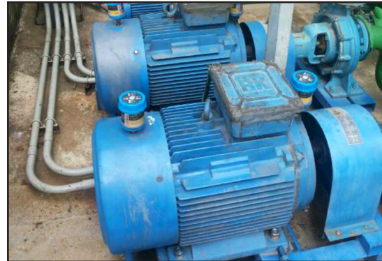
Chesterton's electric motor reliability solution was installed.
